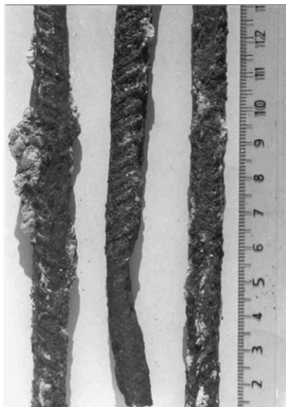
Fig. 4. Parts of a rebar taken from the slab contaminated with chlorides, showing a high degree of corrosion.
